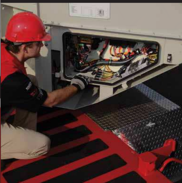
Illuminated upper electrical panel
