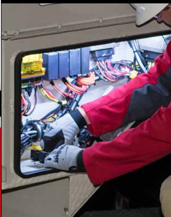
Upper electrical panel
