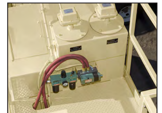
Low-level and high-level switches prevent over-filling of the surge bin.
