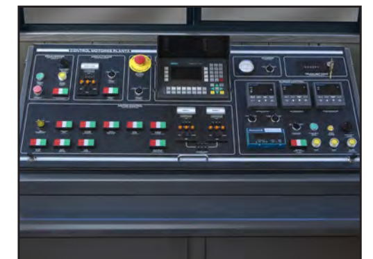
Plant controls are mounted on a centralized control panel.
