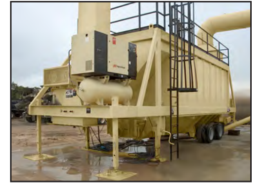
The baghouse includes air compressor, caged ladder and handrails.
