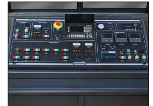
Plant controls are centralized on a control panel located in the control house.
